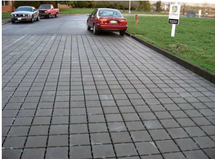
Figure 3. PerVIOUS pavers used in the roadway of a neighborhood development in Wilsonville, OR (Source: Abby Hall, US EPA).
